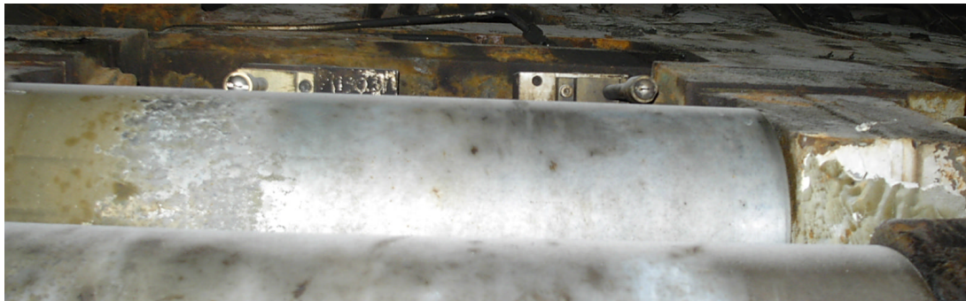
Figure 5 – Misaligned and off position air mist nozzles.
