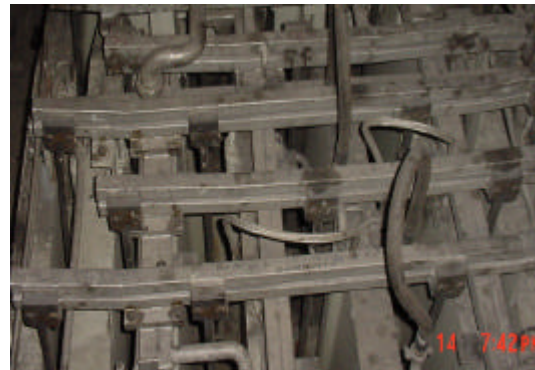
Fig . 10: Square pipe headers carrying Master Cooler SMART type air mist nozzles at HKM/Germany SMS-Demag 2-strand slab caster
