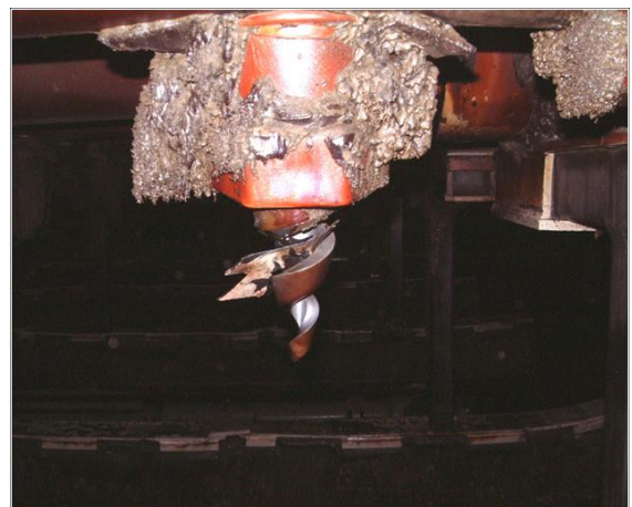
Hydraulic spiral nozzle used in Wet Flue Gas Desulphurization plugged with internal debris
