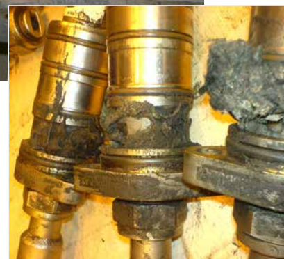
Modulax valves taken out of a badly polluted header. Valve entry ports are completely blocked.
