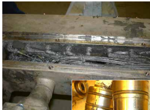
Rear chamber of a Modulax valve header full of emulsion scum
